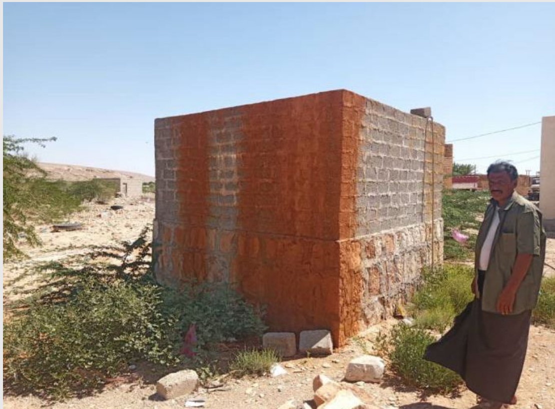
Figure 7: Water tank with iron residues
