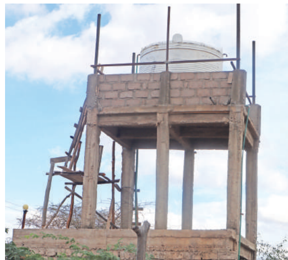
Water storage tanks constructed by the county to provide water for irrigation to the people in Loima, Turkana County. PHOTO/ PSA
